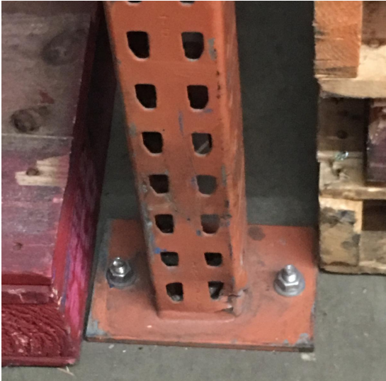
STEP #1 - IDENTIFY DAMAGED RACKING
